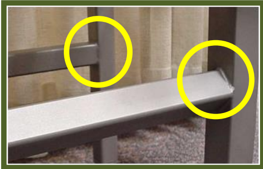
Figure 19. The square tubing on the left will accumulate soil on the flat horizontal surface. By rotating 90°, or using round tubing, flat surfaces are minimized.
