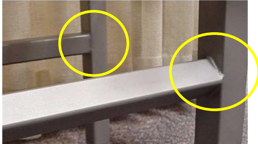
Fig. 19. The square tubing on the left will accumulate soil on the flat horizontal surface. By rotating 90°, or using round tubing, flat surfaces are minimized.
