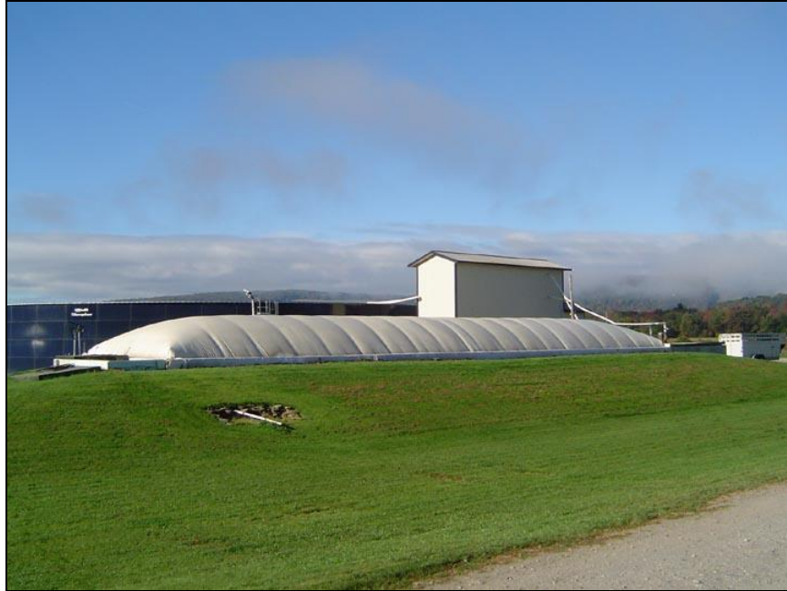
Figure 11. A horizontal plug-flow digester with a flexible top membrane located in Cortland County.
