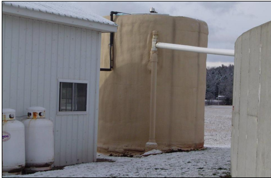
Figure 13. A vertical fixed-film digester located on a 100-cow tie stall farm in the Catskill region of NY
