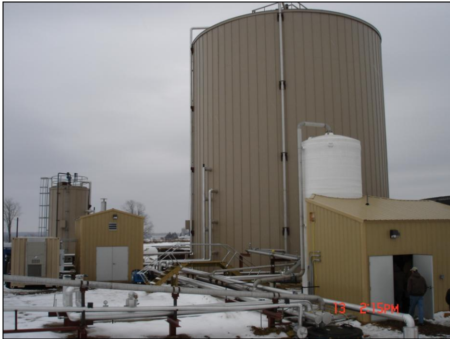
Figure 12. Above-grade complete mix vertical digester on a Wisconsin dairy farm.
